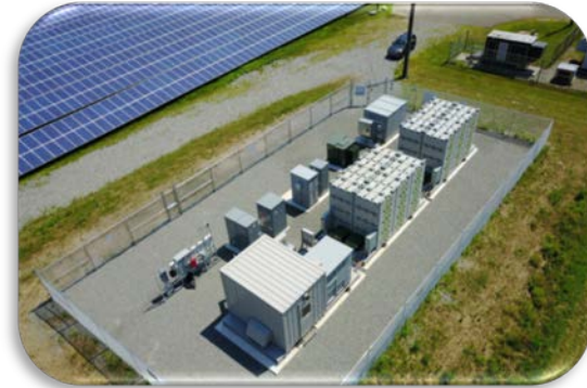
Eos Energy Storage
